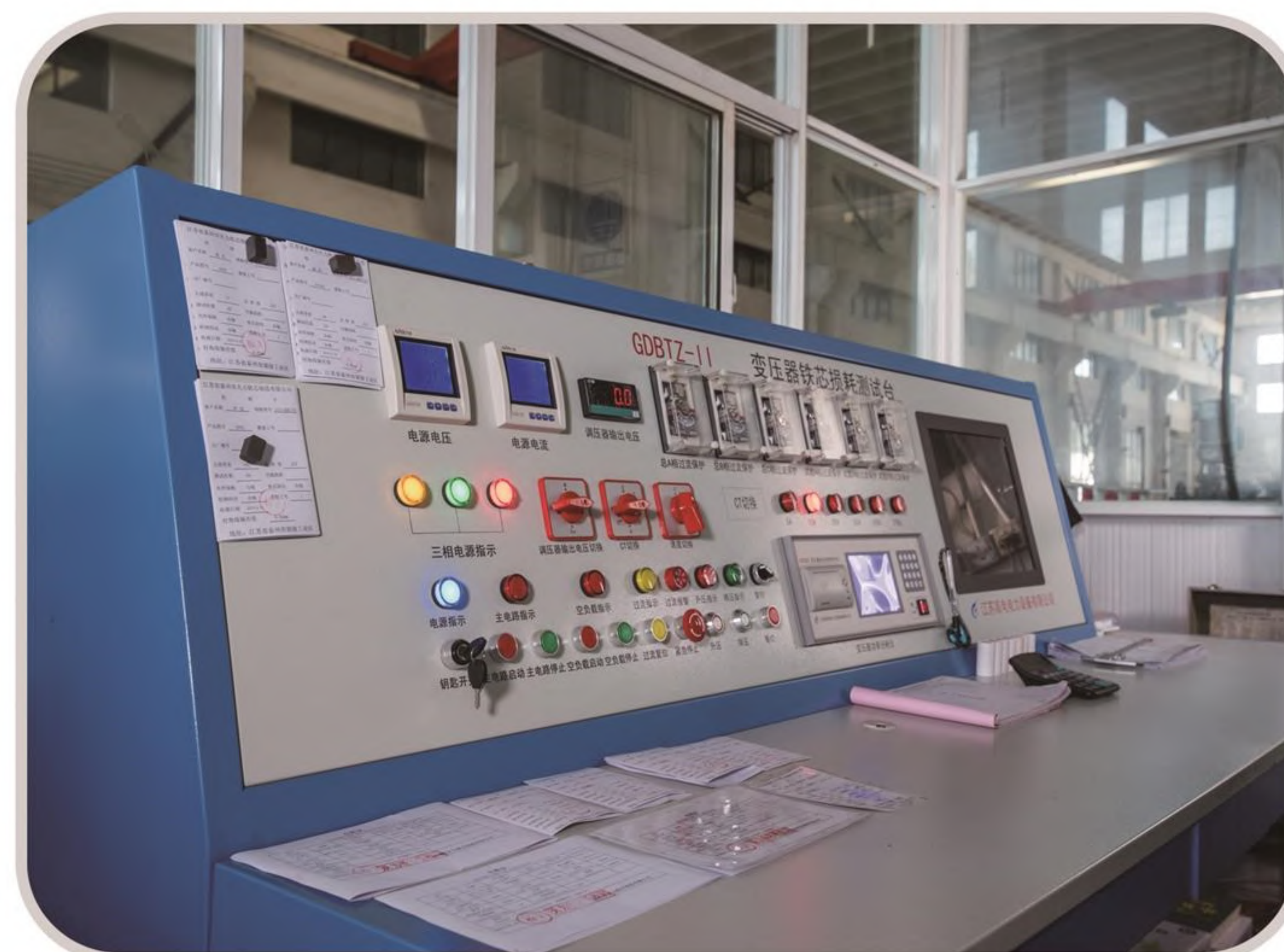
▲ 变压器综合性能测试台 Comprehensive Performance test-bed of transformer
